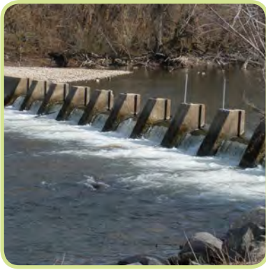
Settlers Diversion, near Ann Morrison Park, is a hazard to floaters.
