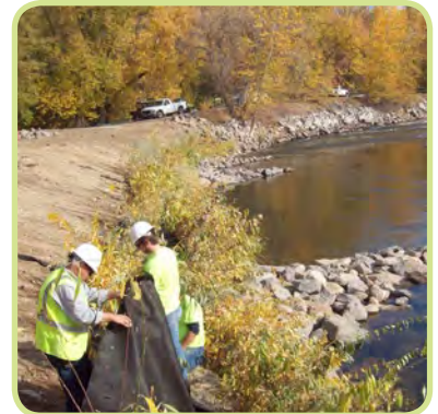
Boise Parks and Recreation crews have developed expertise at constructing river barbs and using bioengineering techniques to protect and restore river banks.
