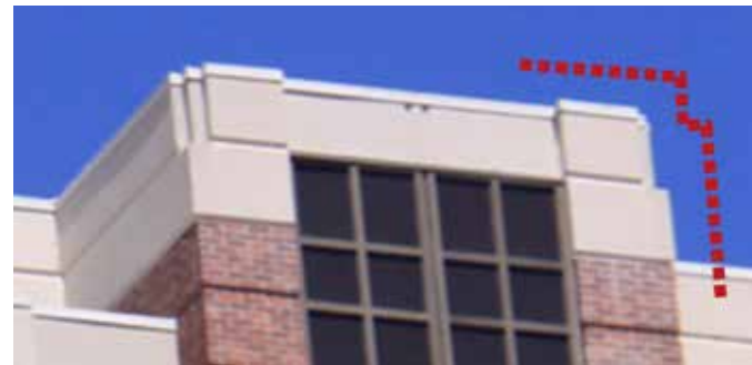
St. Luke's uses a combination of reliefs, steps, and materials to create a stepped pediment.
