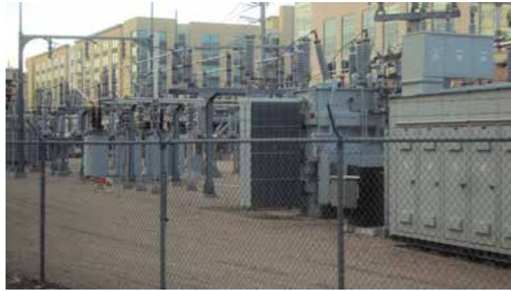
Grove Street Substation.
