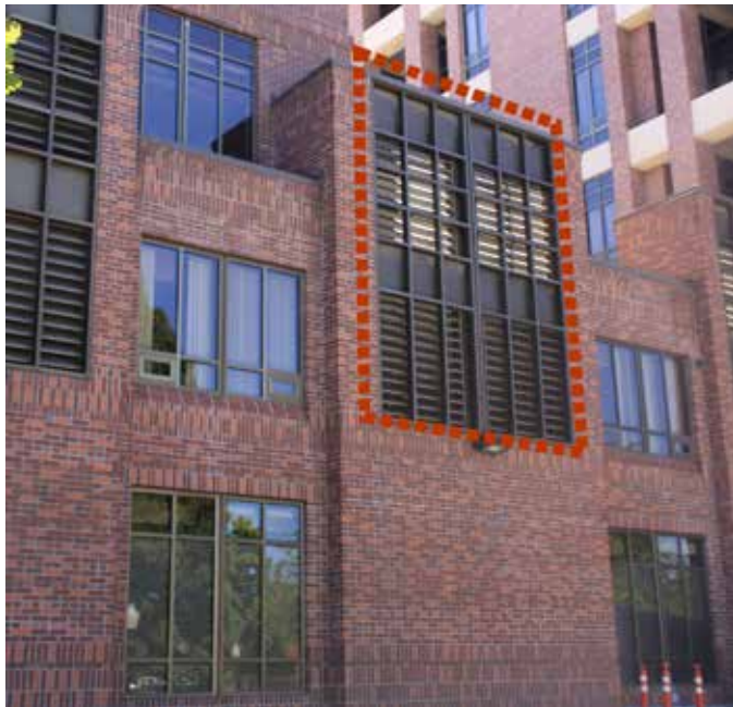
Mechanical grilles at St. Luke's Boise match adjacent window color. Grilles are divided by vertical and horizontal mullions that match the vocabulary of the adjacent glazing systems.
