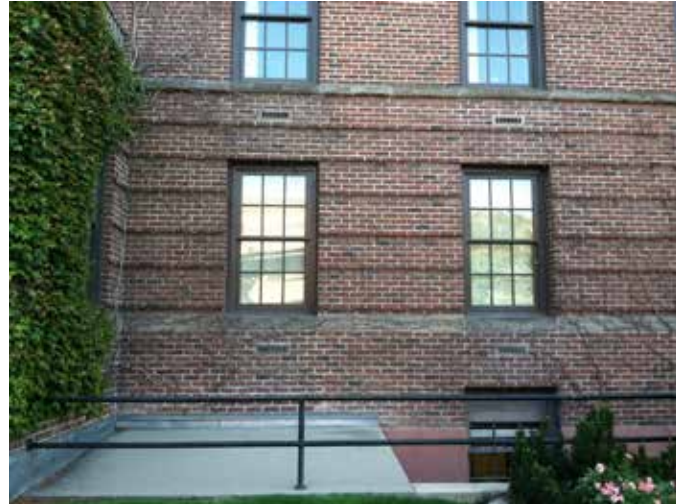
Use of reveals and coursing in the brick to create a base at the 1927 St. Luke's Boise hospital.
