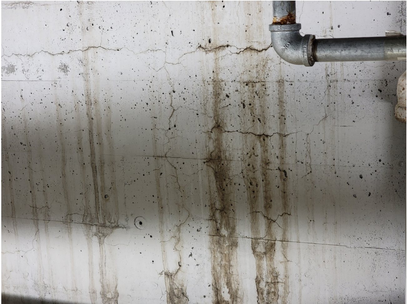
Figure 10: Interior Pool Wall – Minor Cracking
