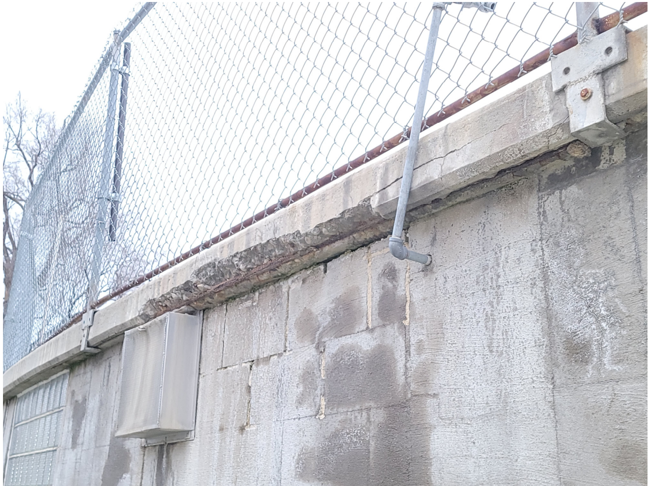
Figure 6: Deck slab – Bottom of Deck Deterioration due to ASR/ Exposed Rebar
