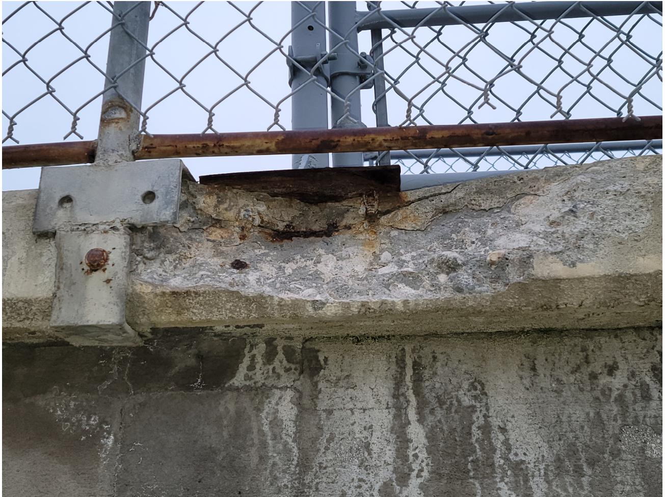
Figure 8: Deck slab – ASR/Deck Spalling Under Fence Base Plate / Exposed Anchor
