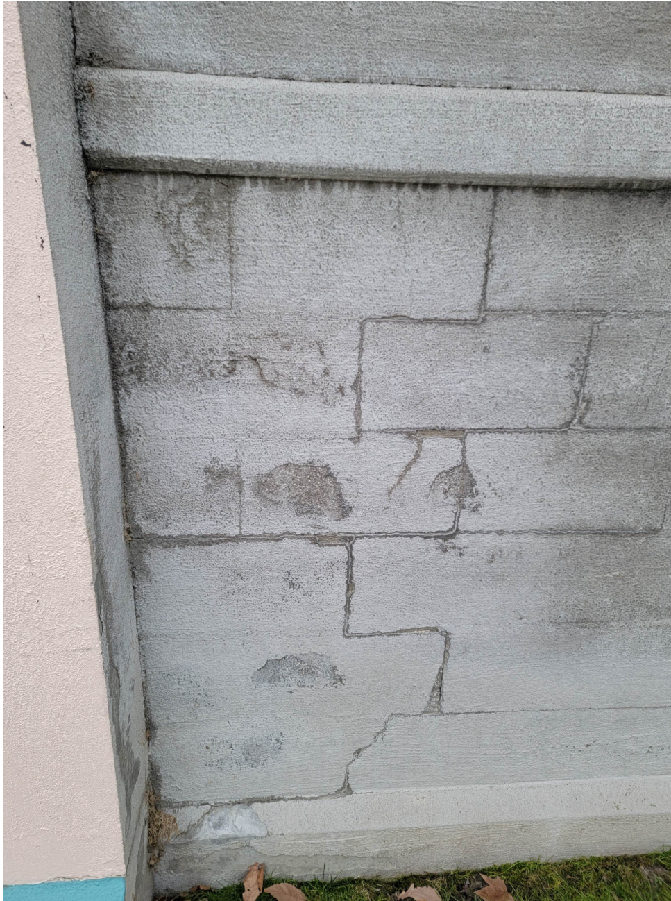
Figure 11: Outer CMU Wall – Minor Cracking
