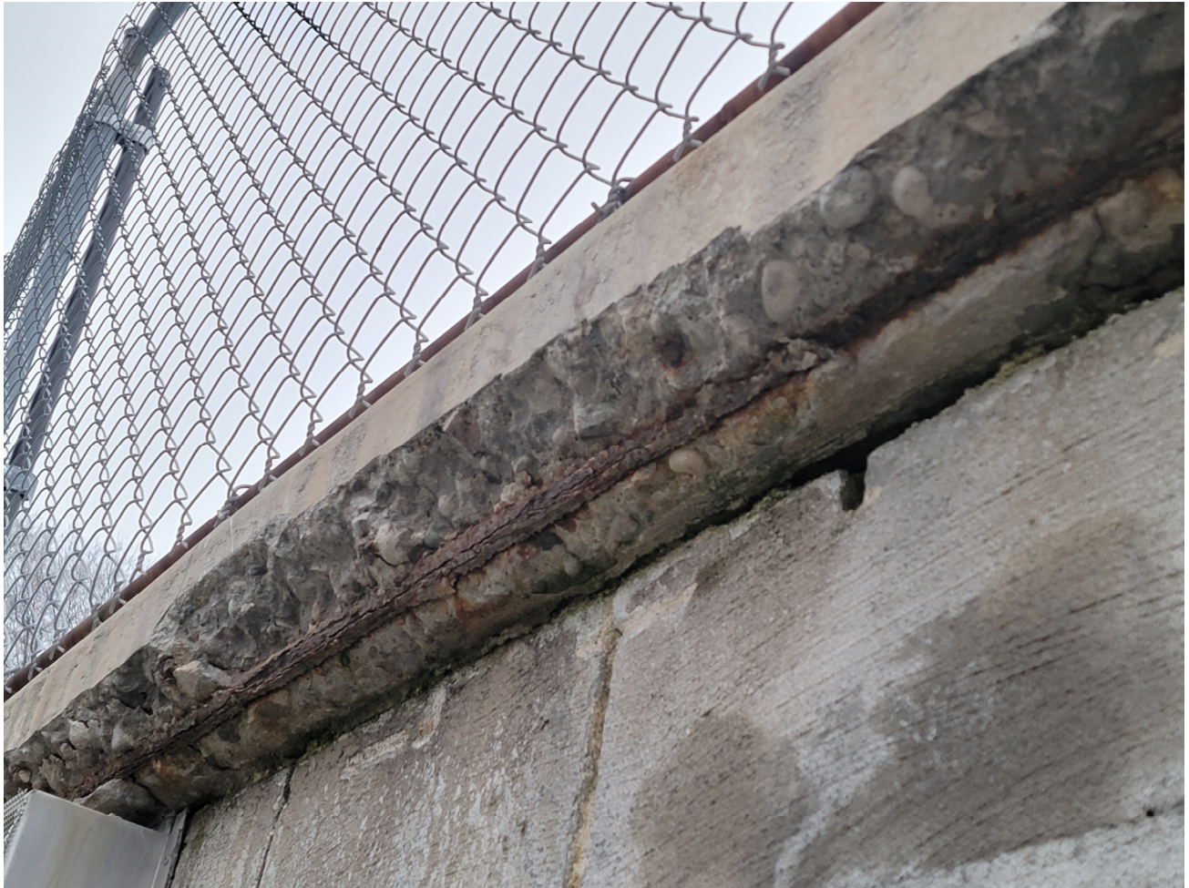
Figure 7: Deck slab –Damaged Concrete / Exposed Rebar
