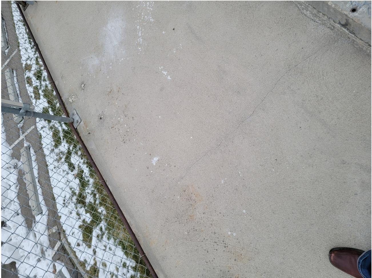
Figure 5: Deck slab - Minor Topside Cracking
