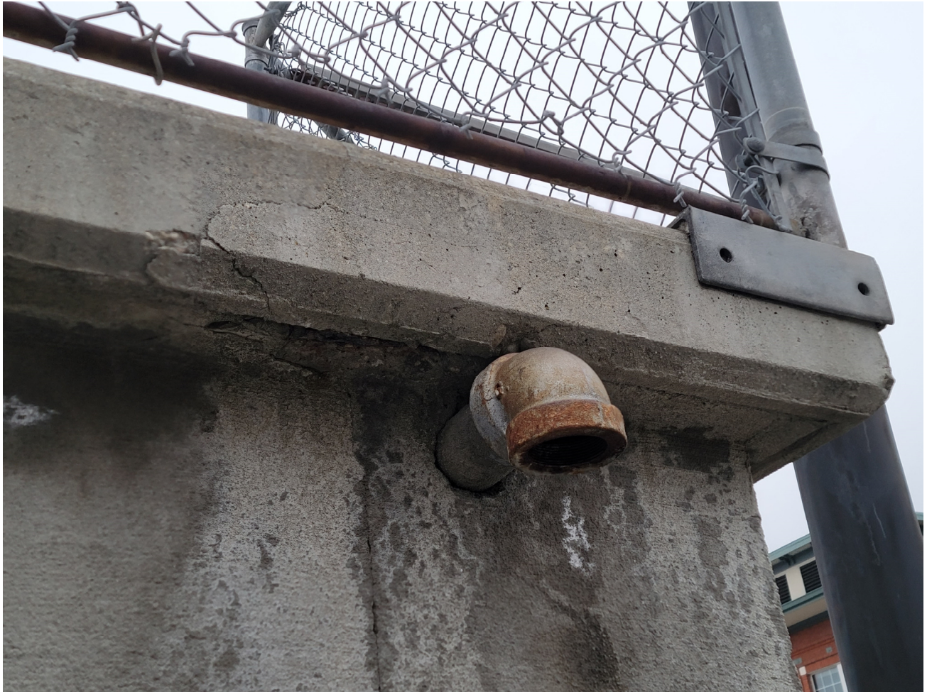
Figure 9: Deck slab – Minor Cracking at Edge of Top Deck
