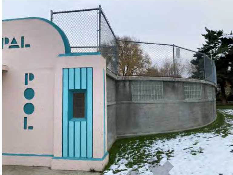
Exterior façade – showing deteriorating/aging skim coat on the CMU block. Chain-link fencing shown above.
