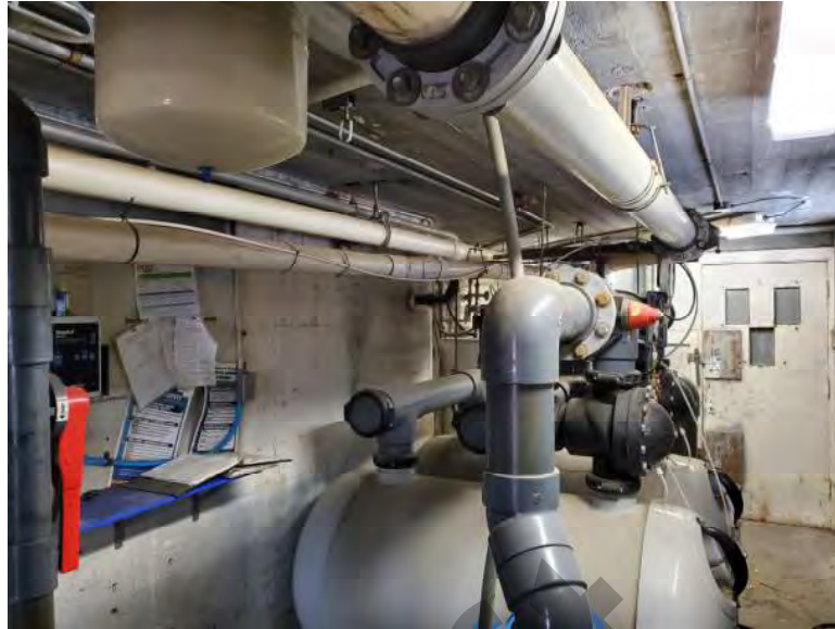
Piping for pool systems.
