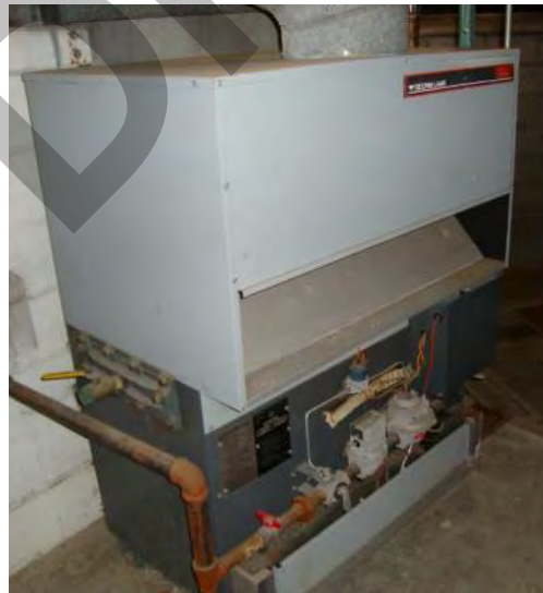
Lowell Pool Heater.
