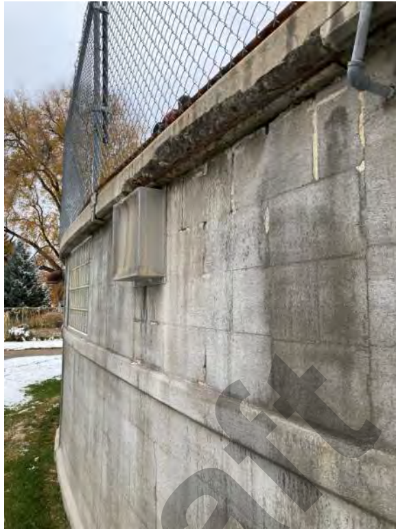
Concrete cracking and exposed rebar at deck edge.
