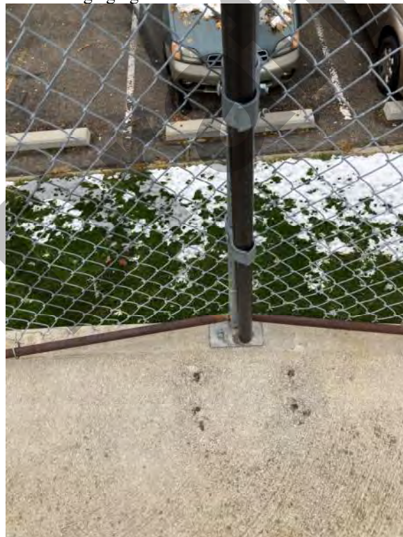
Rust showing at bottom of fence piping.
