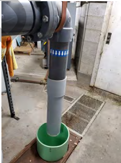
Pool systems drain through grating.
