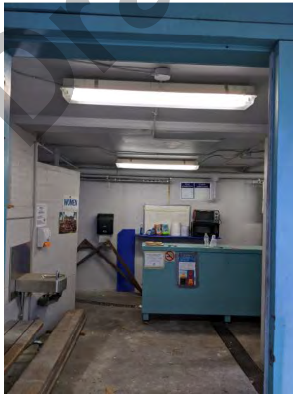
Typical Interior Light Fixture.
