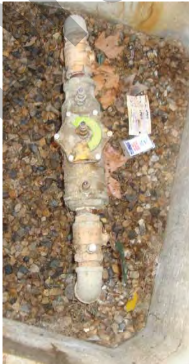
Lowell Water Service Backflow Preventer.
