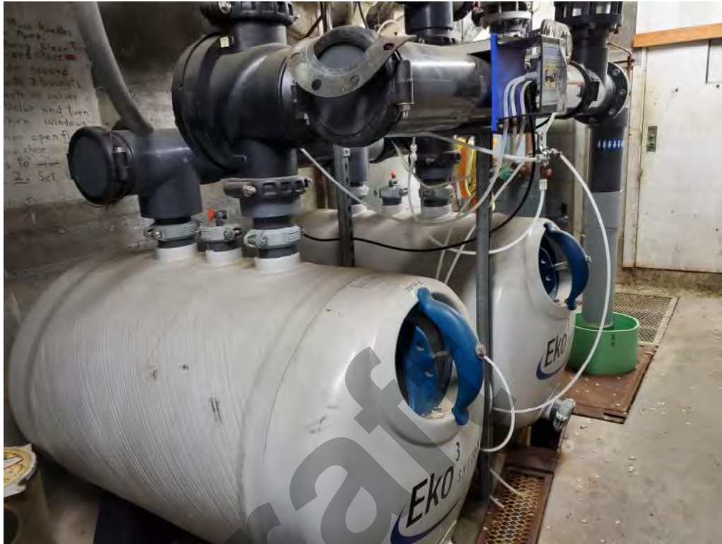
Pool systems tanks.
