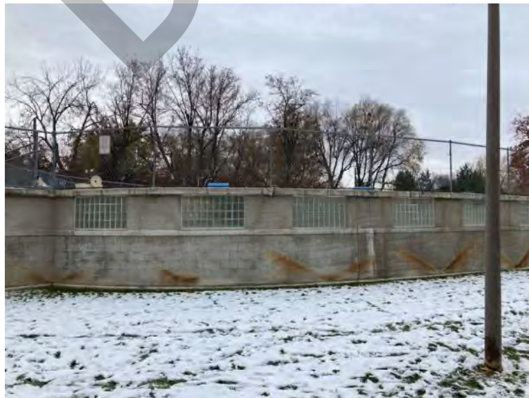
Exterior façade – showing water staining and deteriorating/aging skim coat on the CMU block. Chain-link fencing shown above.
