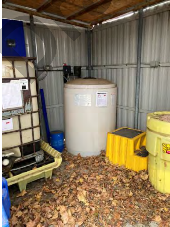
Inside of pool equipment storage shed at far west side of facility.
