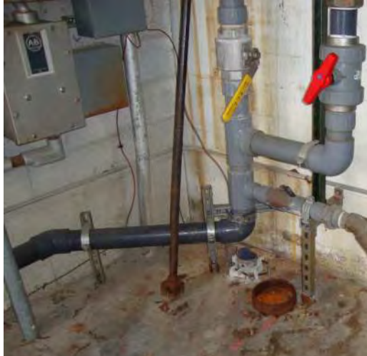
South Domestic Water Service Entrance (Section of Underground Piping Replaced with Plastic).
