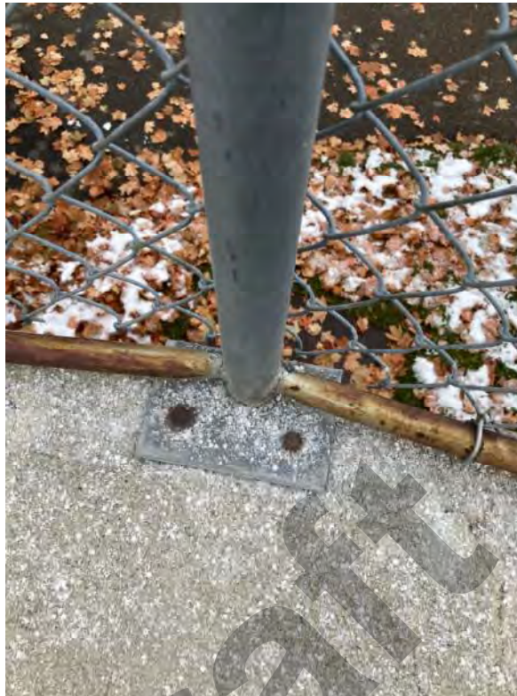
Rusted fence piping and bolt connections shown at fencing.
