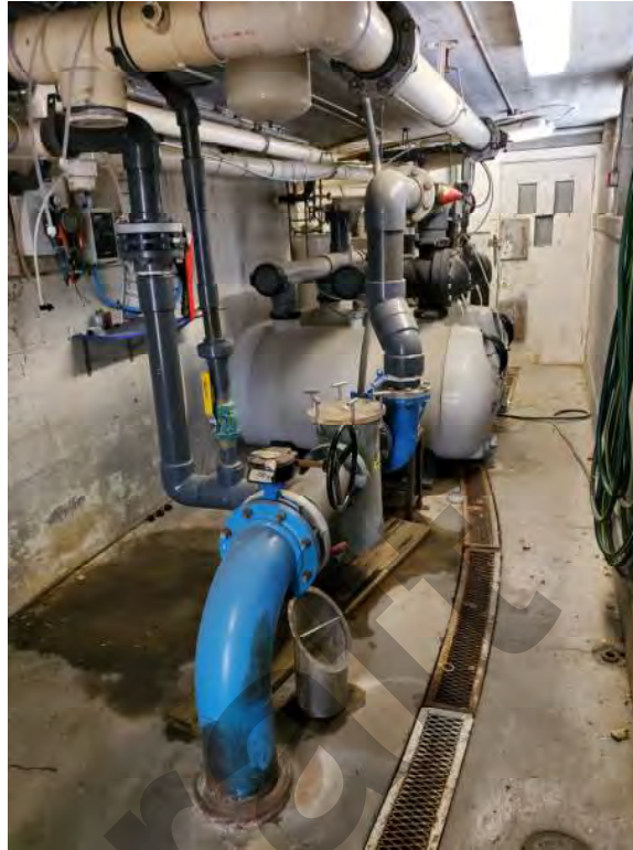
Pool equipment room.
