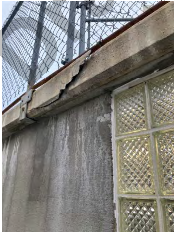
Concrete cracking at deck edge.
