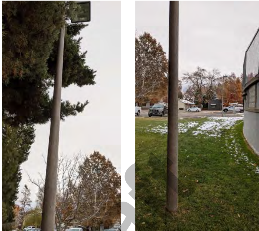
Exterior Pole Light.
