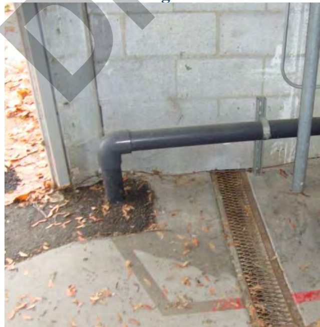
South Domestic Water Service Entrance.
