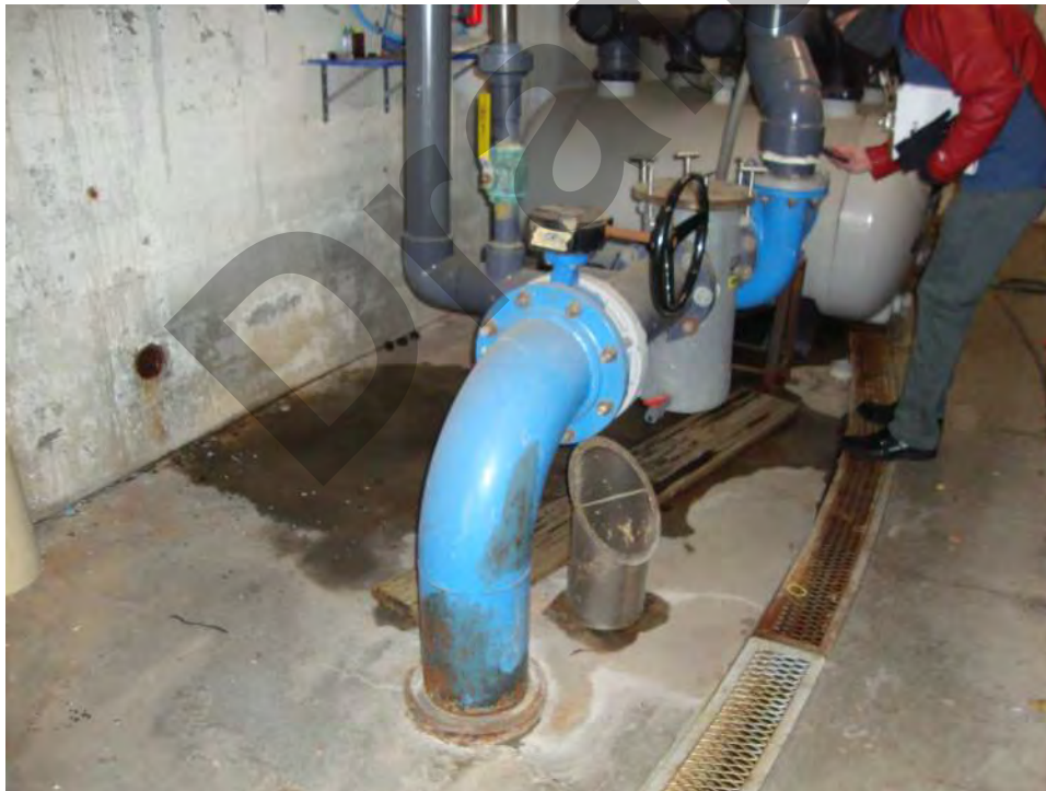
Underground Cast Iron Piping from the Pool Main Drain to the Circ Pump.
