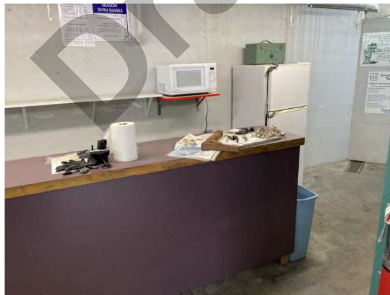
Entry desk – showing plastic laminate peeling.
