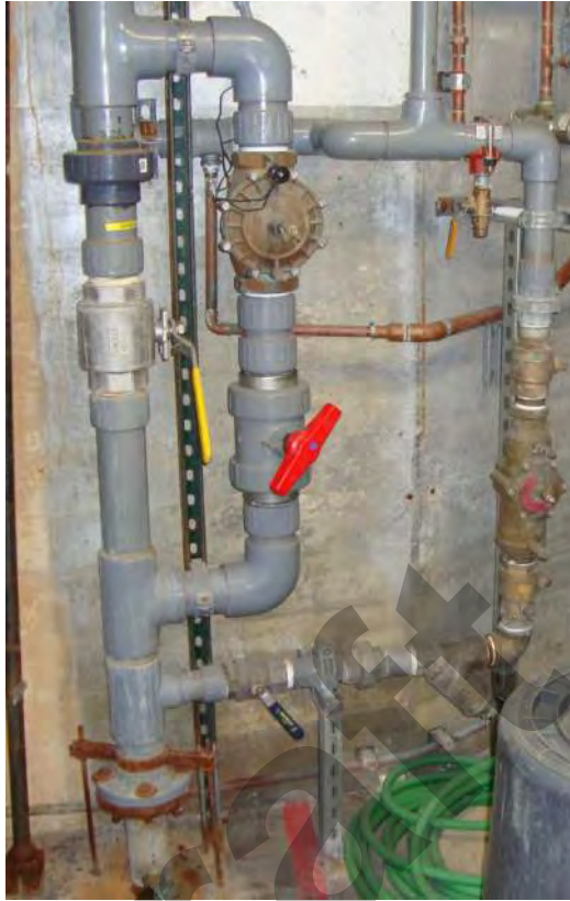
Lowell Domestic Water Service Entrance.
