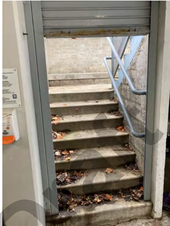
Main building entry/egress stair - shows roll up door.
