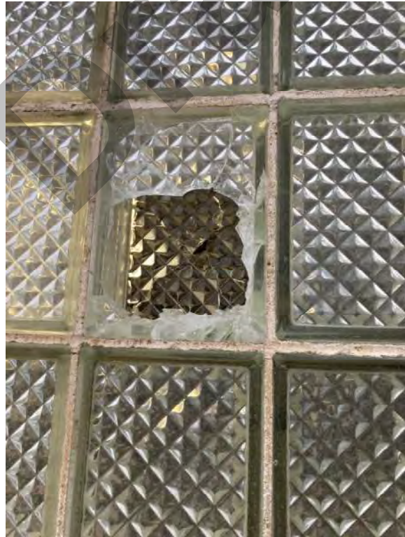
Glass block cracked and damaged.
