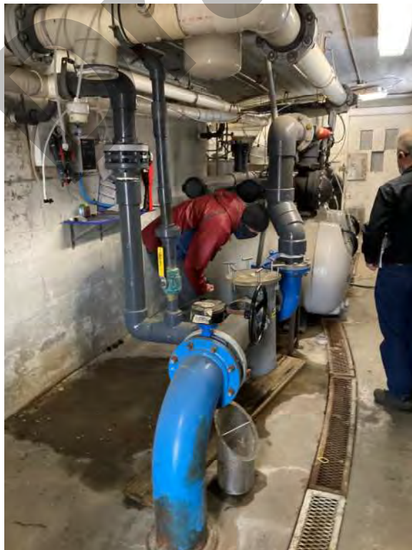
Pool pump room. Shows rusted floor grating.
