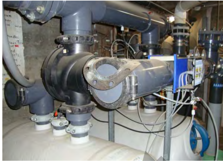
Lowell Pool Filtration & Water Treatment.
