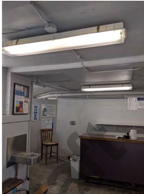
Typical Interior Light Fixture.
